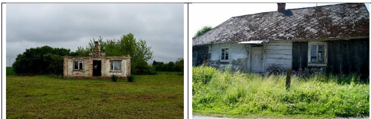
Plate 2. Examples of the deterioration of residential buildings in disappearing villages of the Lublin region.
